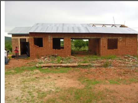
Admin Block with tin roof. This will be a store and office space.
